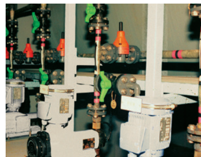
Ferric chloride pumping in purification station.
