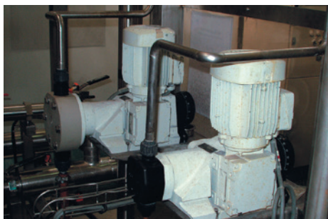
Metering of soda and acid.
