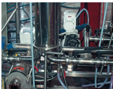
Pump on filtering pallet (wine production).
